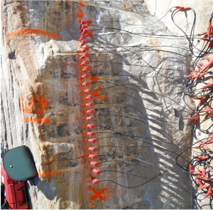
Figure 5.14: Shot area 15 was analyzed using an MASW geophone array of 1.83 meters (6'). The gathered data were specific to the 1.52 meters (5') wide section of stone blasted in shot 15.
