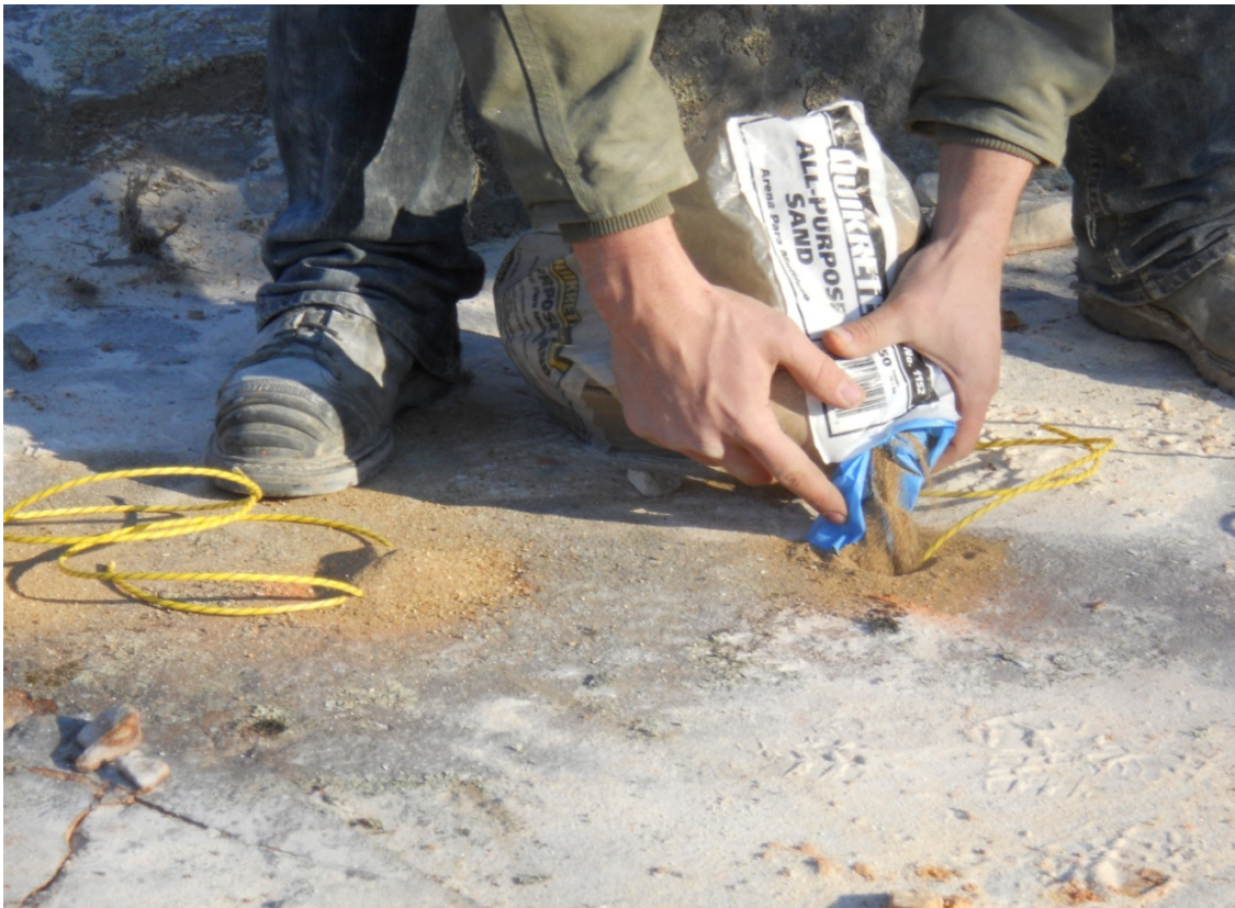
Figure 5.6: Sand was used as stemming media to confine the explosives in the boreholes.
