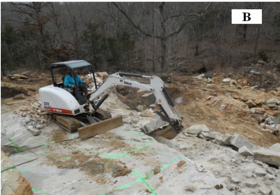
Figure 5.7: Machinery aided in excavating the blasted stone. Some of the equipment used included: A) Caterpillar 920 fork lift; B) Bobcat 331 mini excavator.
